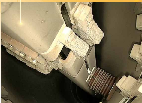
Detect braids deterioration
