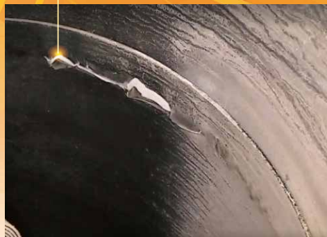
See where bellows cracks are forming
